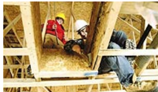
Students Kevin Heyerhoff, 17, left, and Jason Rousseau, 18, install an attic hatch in a house as part of the Construction Focus Program yesterday. (Blair Gable/SUN)
